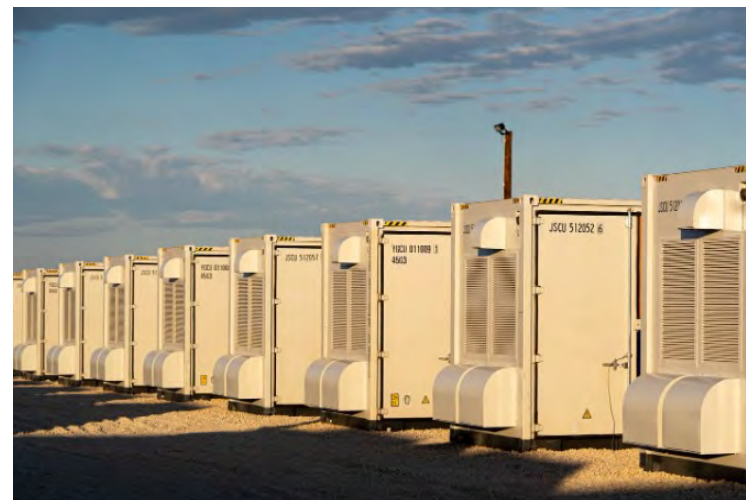
Jupiter Power’s Crossett battery project in Crane County, Texas (Jupiter Power)
